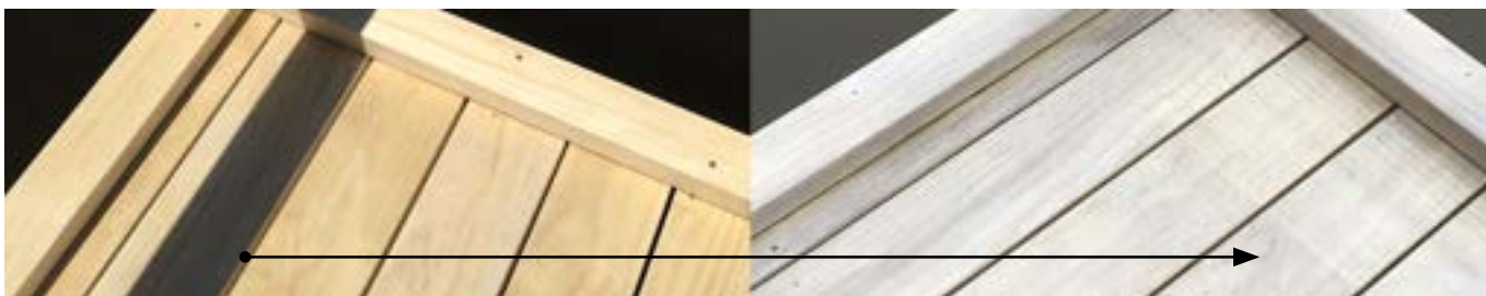
Natural greying of Accoya decking over time
