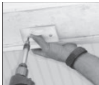
3. Fasten one plate (two halves), edges down, to the beam above. Using a plumb tool, find and mark bottom position on floor.
